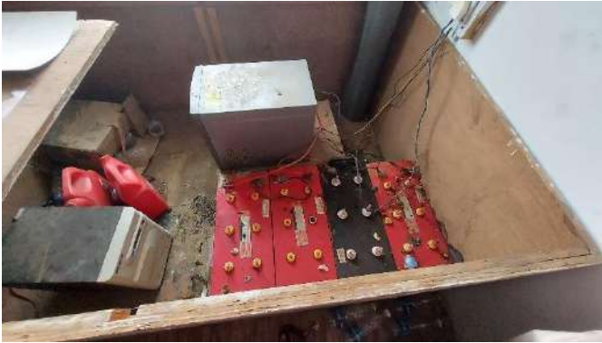
Figure 14 - Placement of battery is in danger
