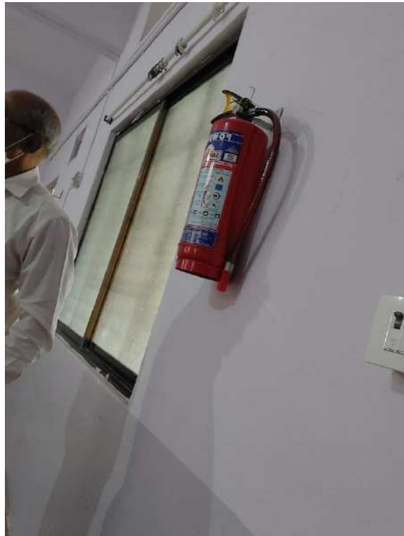
Figure 20- Need ready access to fire extinguisher.
