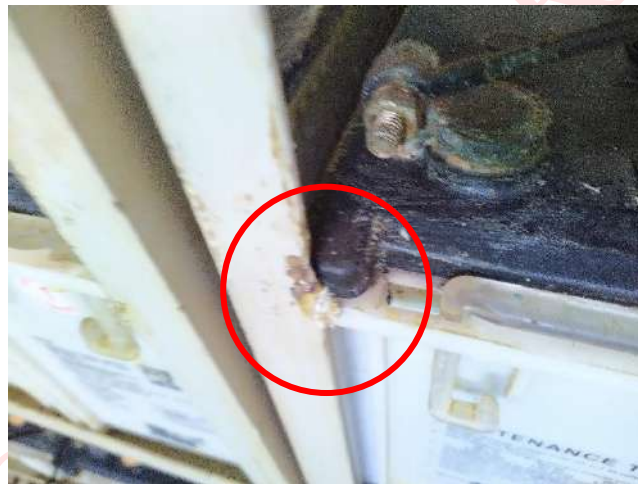
Figure 16- Galvanic reaction causing damage to battery life.
