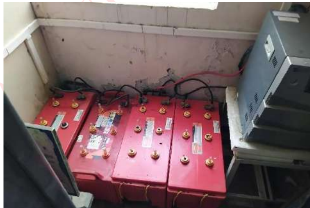
Figure 15 - Placement of battery without ventilation
