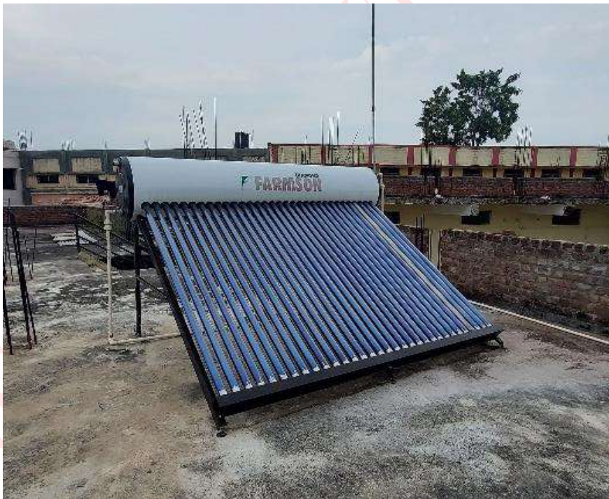
Figure 10 - Solar water heater
