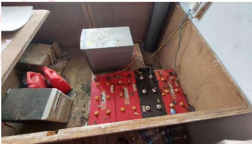
Figure 14 - batterieus in enclosed box.
