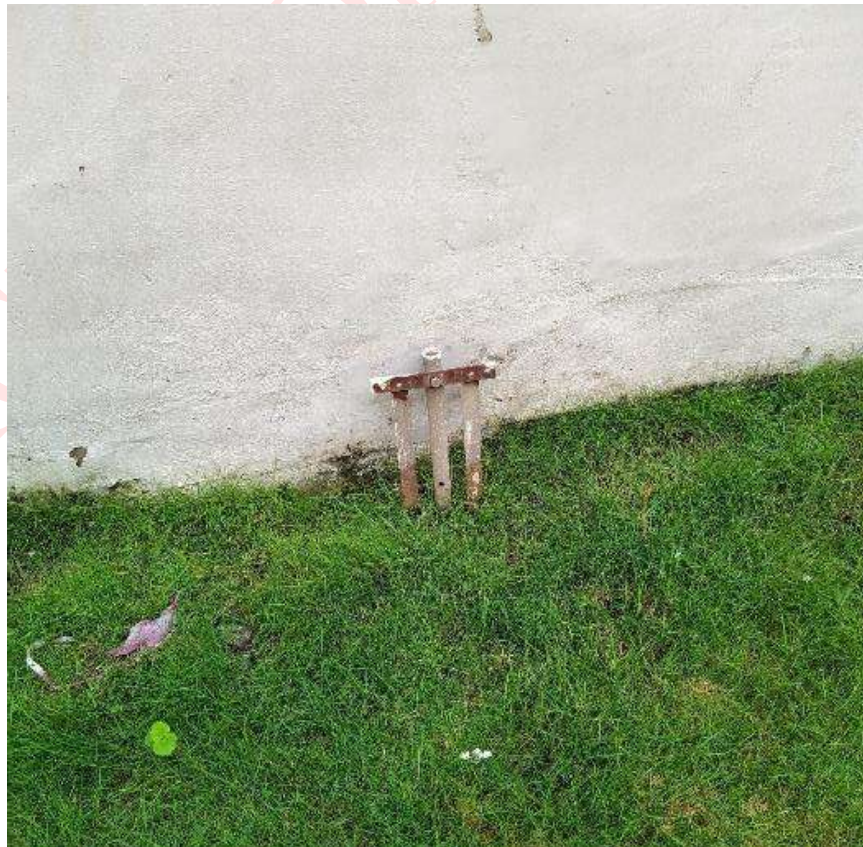
Figure 18 - Safety, electrical earthing compliance
