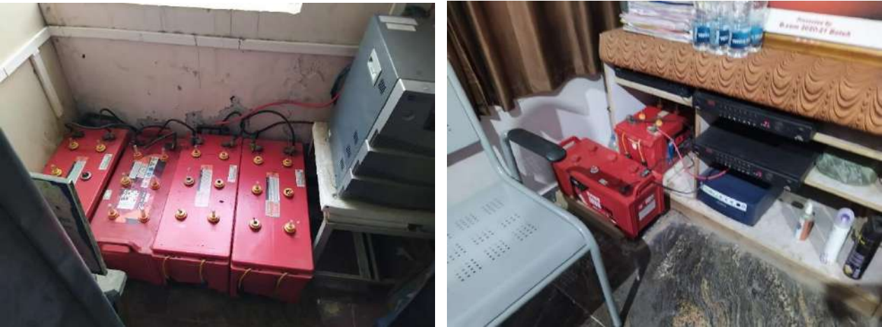
Figure 15- Battery placement, Need cross ventilation.
