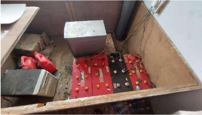
Figure 14 - Placement of battery is in danger
