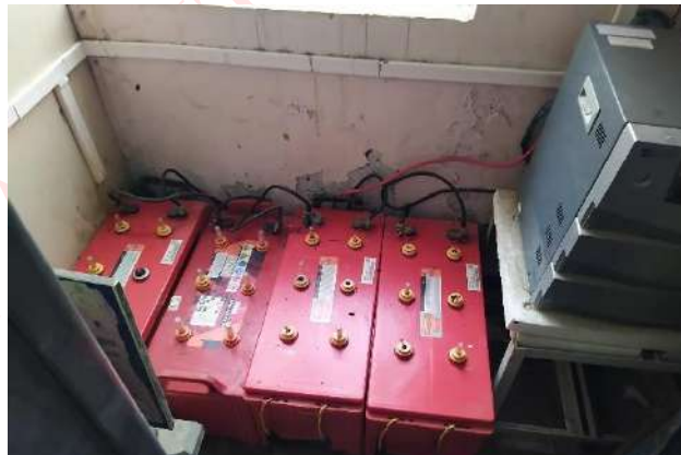
Figure 15 - Placement of battery without ventilation
