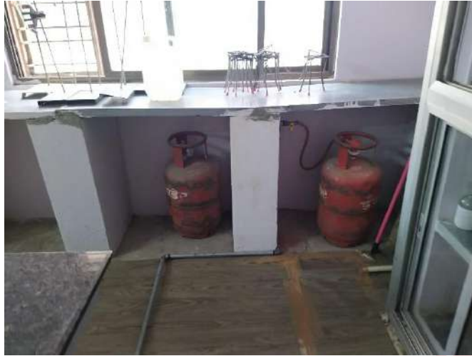
Figure 24- Placement of LPG cylinders in wrong location.
