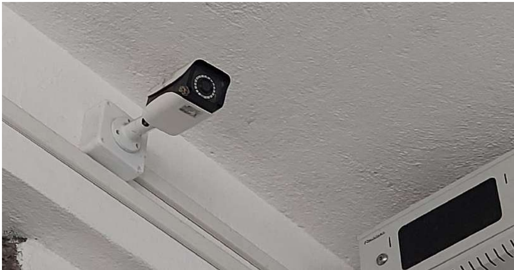
Figure 11- CCTV for security
